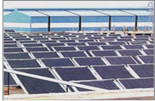
Fig 3.17: Solar Panels to trap solar energy
